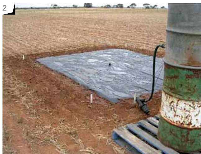
Photo 2: Completed pond showing header tank, in-line filter and wetted area covered in plastic sheet, the edges of which were placed in the trench before back filling with soil.
