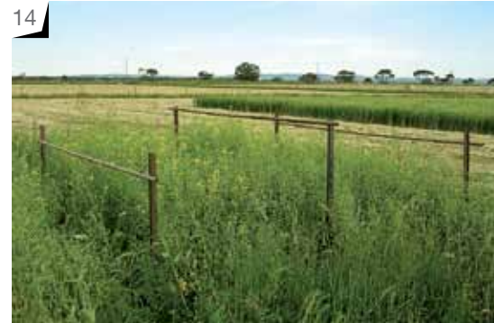
PHOTO 14: Rain-exclusion tent frame: consists of six star-posts with three pipes or box section wired between them. Posts are positioned to support a 3 x 3m tent.
